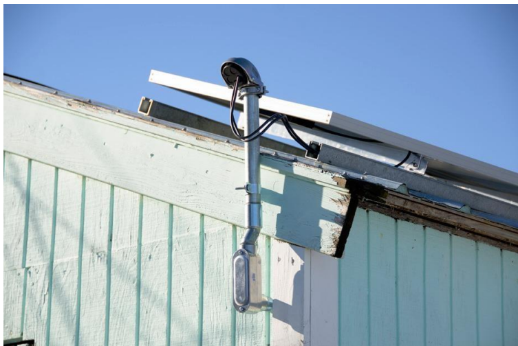
Figure 4.26: Flush mount solar array with cable entry through electrical service entrance and then through the wall of the health facility. Photo courtesy of FGL/IM-PAHO and SELF.
