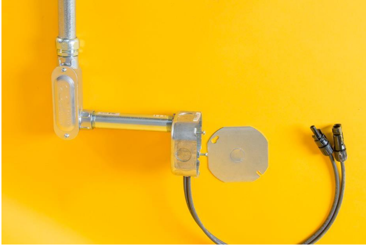
Figure 4.27: Example of exterior conduit with conduit body and short conduit passing through the wall where the solar array cable is in the health facility. Photo courtesy of FGL/IM-PAHO and SELF.
