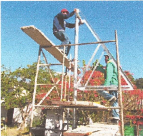
Figure A.4: The scaffold provides a safe, secure and level work surface. However this scaffold has an unsafe work platform.
