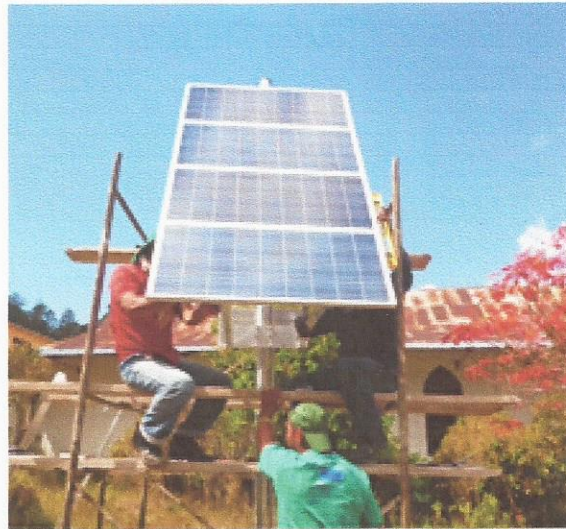
Figure A.5: Solar modules would be difficult and more risky to position with a ladder.
