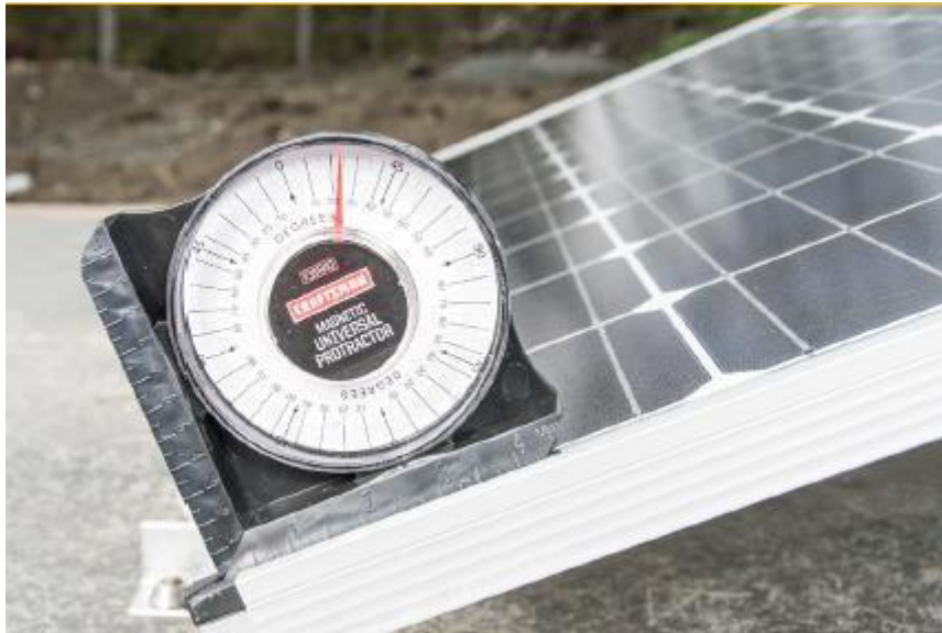
Figure 4.15: An inclinometer (protractor) can be used to confirm the tilt angle is correct. Photo courtesy of FGL/IM-PAHO and SELF.
