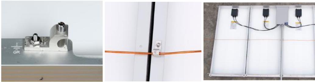
Figure 4.10: Solar module ground lug, fastener and ground wires connected. Photos courtesy of FGL/IM-PAHO and SELF.
